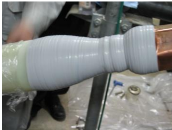
Figure 20 well installed cable termination
