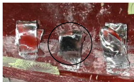
Fig 17. The PD location of the dissection transformer in Case 1
