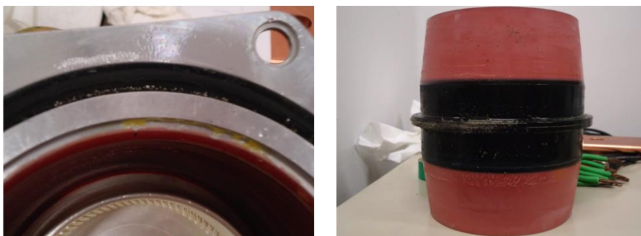
Fig. 13 busbar socket with pollutants
