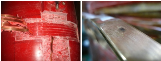
(a) Dissection (b) Defect on conductor
