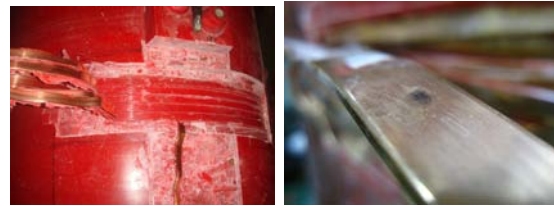
(a) Dissection (b) Defect on conductor
