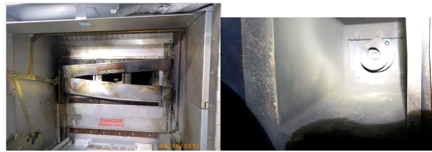
(a) inside panel (b) inside bushing
